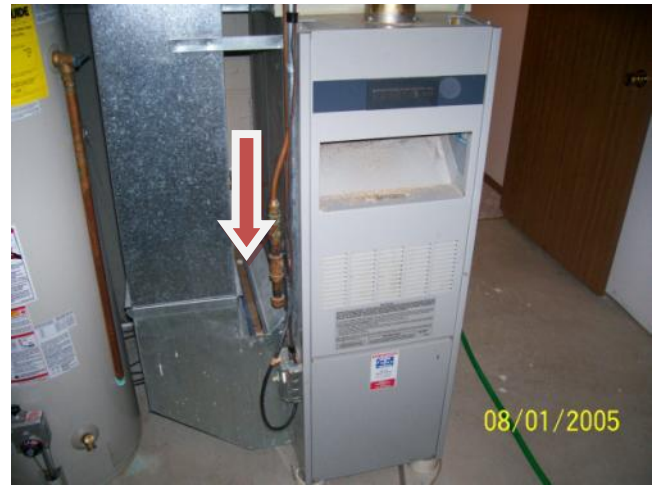
Furnace filter location
